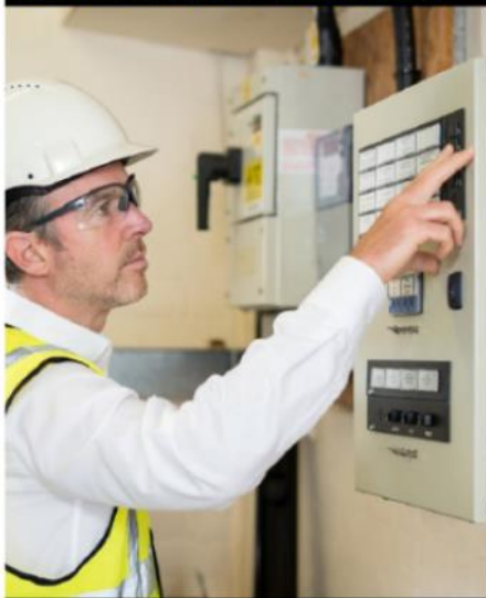
Alarm annunciator panel – Image: Omniflex
